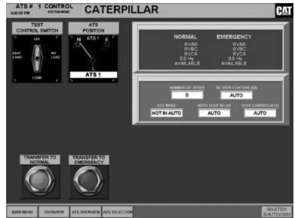
Screenshot of ATS operating parameters on Cat Switchgear HMI.
